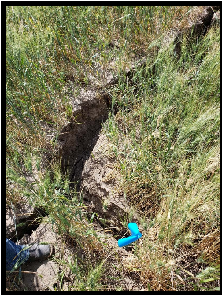
Subsidence occurred along portions of the pipeline in the project area.
