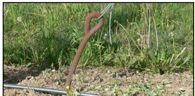
Figure 2. Steel anchors bend above ground when not in line with the pull of the wire. Plan ahead to install steel anchors properly into undisturbed soil. (Photo: Hugh Fraser)
